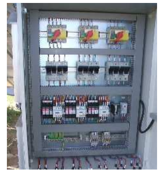
Interior of the above unit
